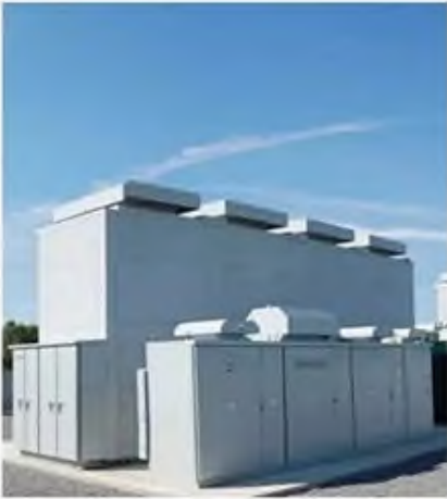
Industrial energy storage
