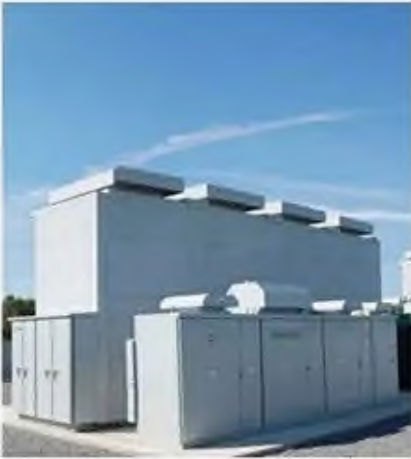
Industrial energy storage
