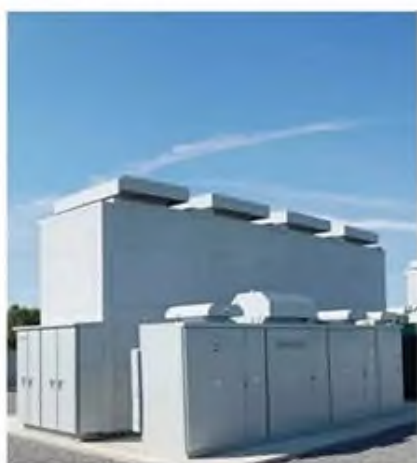
Industrial energy storage
