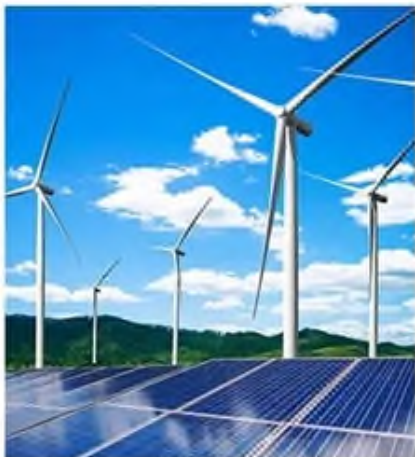
Solar power station
