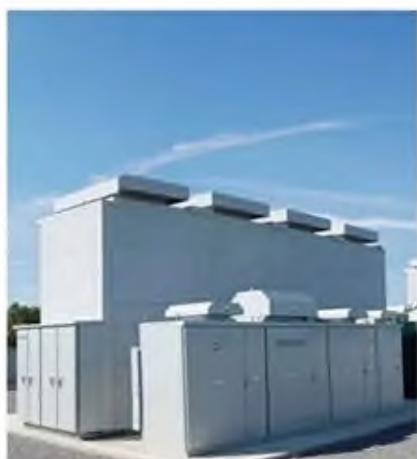
Industrial energy storage
