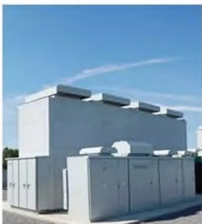
Industrial energy storage
